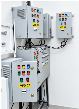
Energy Monitoring Panels
